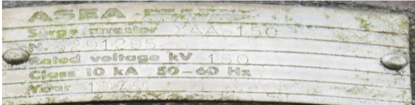
Gambar 2. Nameplate Lightning Arrester (LA) Bay Darajat #1
